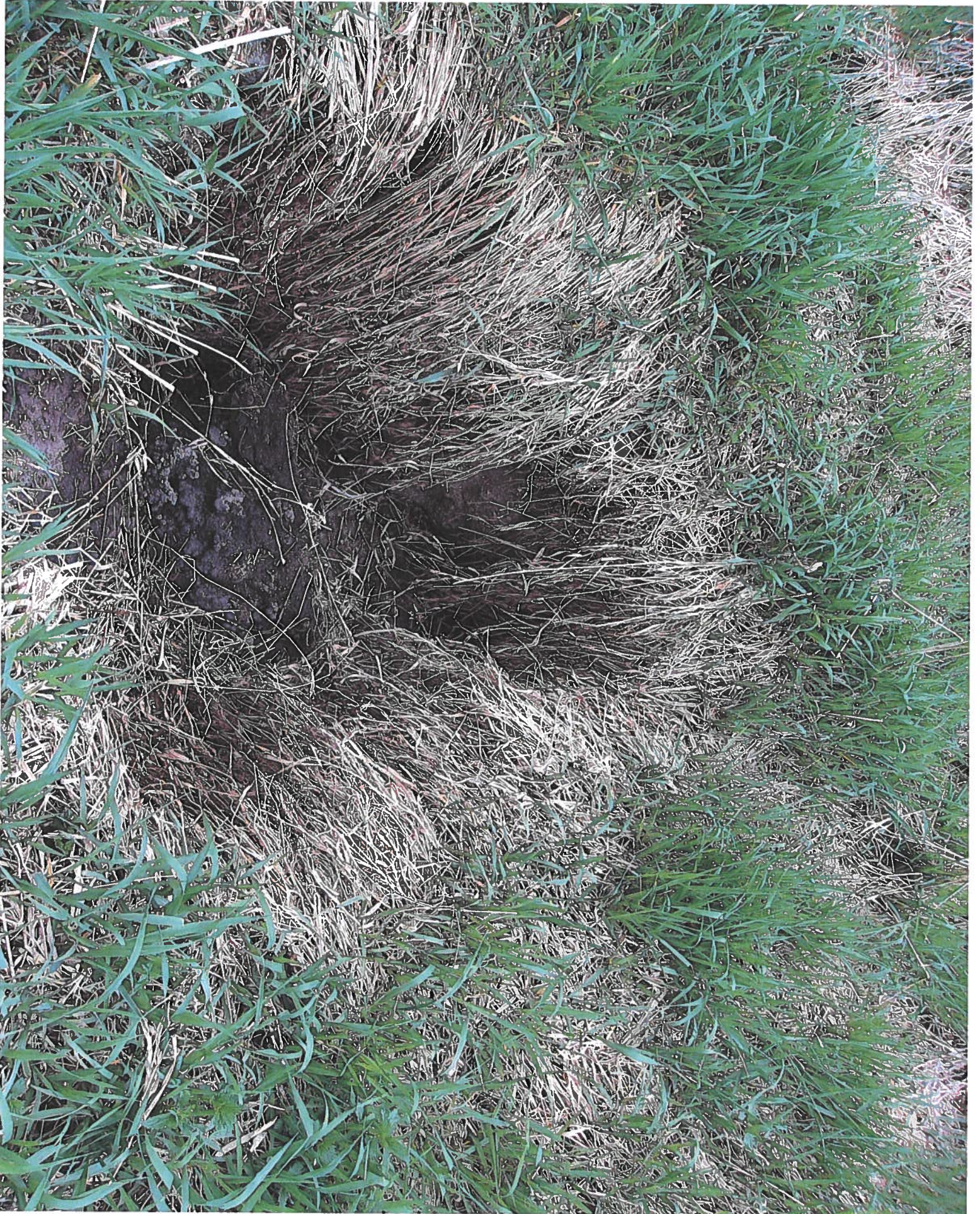
WATER ERODING CONC. ENCASUREMENT @ HEADWALL
