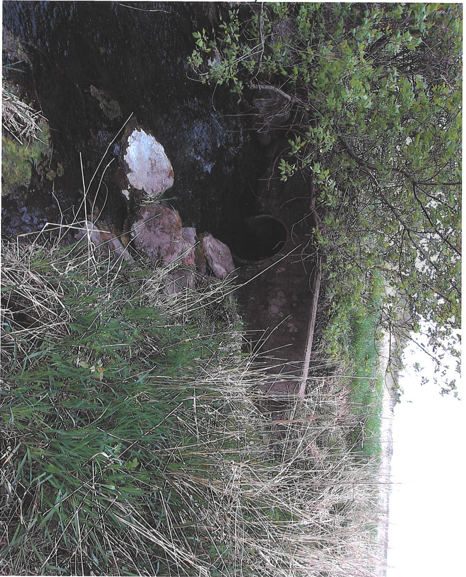
HEADWALL IS FUNCTIONING WELL, HAS LEAK @ BOTTOM TILE.
